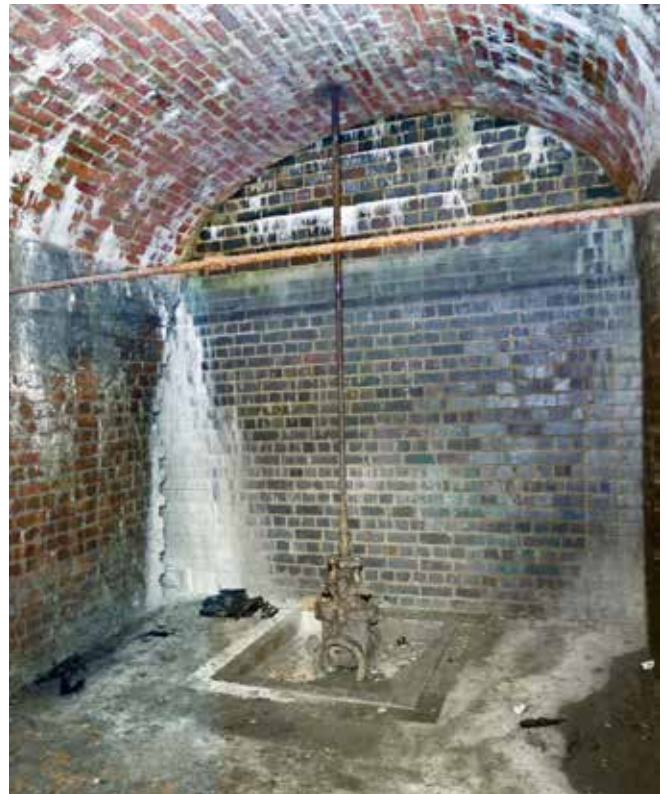
The rebuilt end wall and drainage (?) valve and spindle in one of the middle chambers
